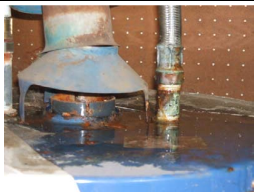
Check Water Heaters for Leaks
